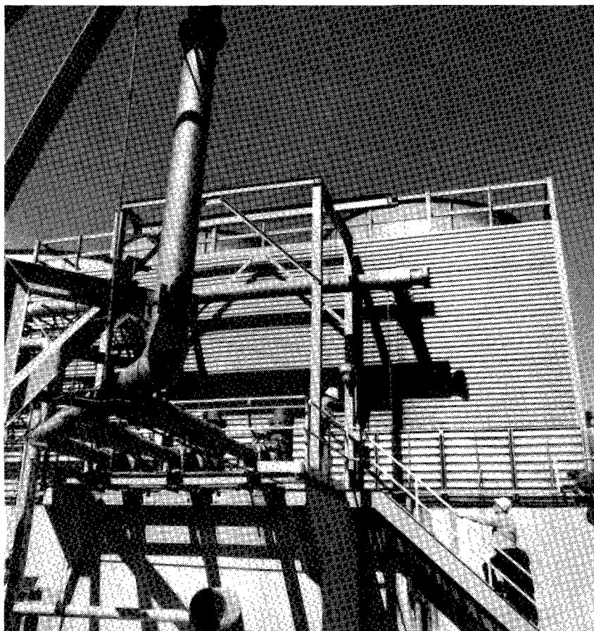
FIG. 1. Biological cooling tower shown under construction at Lever's Edgewater, N.J., plant. Piping in left foreground supplies water from cooling tower to edible process department.
